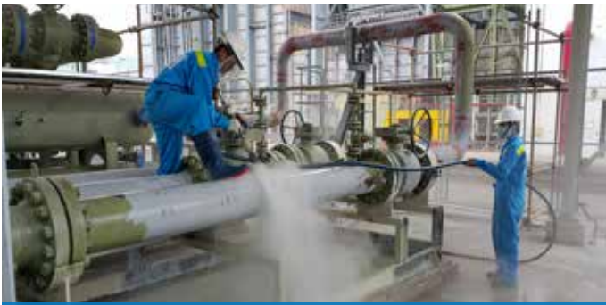
PHU MY POWER PLANT GAS DISTRIBUTION
