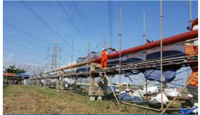
PHU MY GAS PIPELINES
