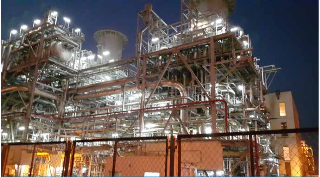
PHU MY POWER PLANT
