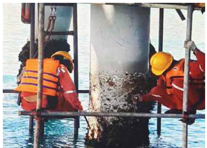
JETTY TO BE CLEANED OF BARNACLES
