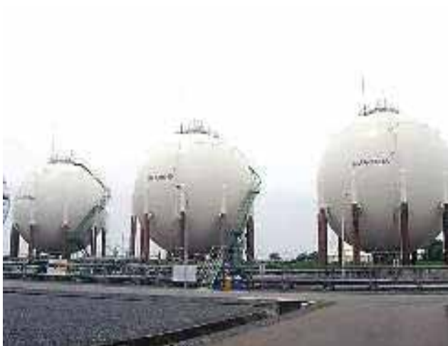
PAINT GAS SPHERE TANKS
