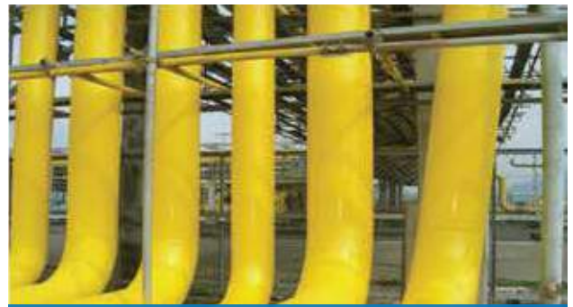
SOUTH EAST GAS DISTRIBUTION
